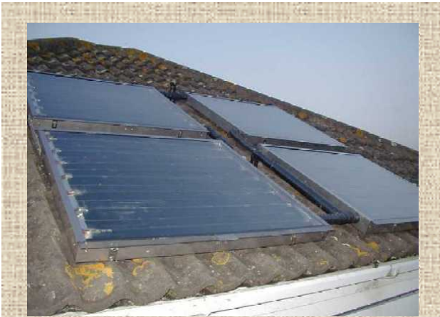
four flat-plate panels installed on a private house in Lincolnshire. The panels are approximately one square metre each, making them easy to transport, and to lift onto the roof.
