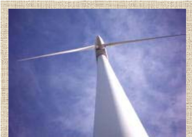
one of two large turbines at Ecotech, at Swaffham, Norfolk. Its capacity is 1.5MW, enough to power 1,100 homes. It was installed by Ecotricity, and you can visit and climb to a viewing platform behind the blades.
